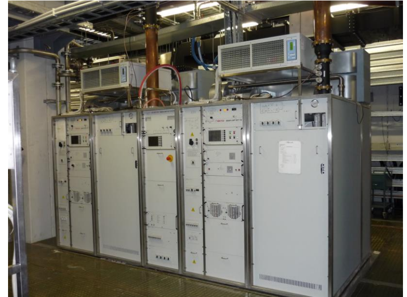
150 kW twin I.O.T.s based transmitter.
